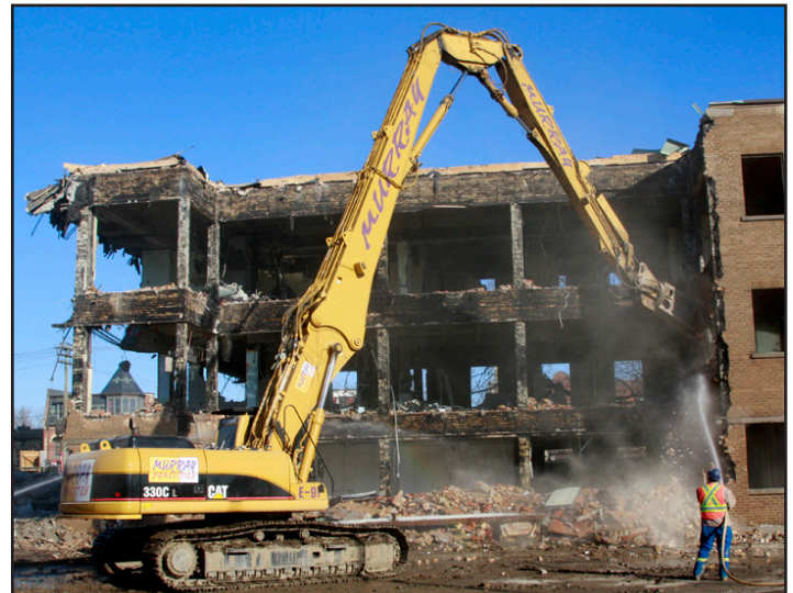
March 10, 2010: A crew member sprays water to minimize dust as heavy machinery tears into the CAMH administration building on Queen St. W.
